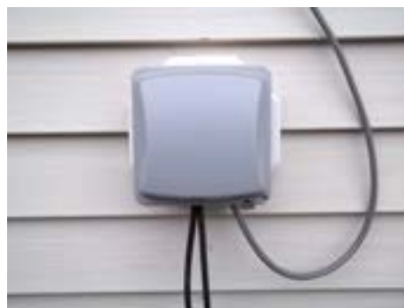
Photo 3. Plastic enclosure, purchased from a big-box store, makes a neat entryway for cables.
