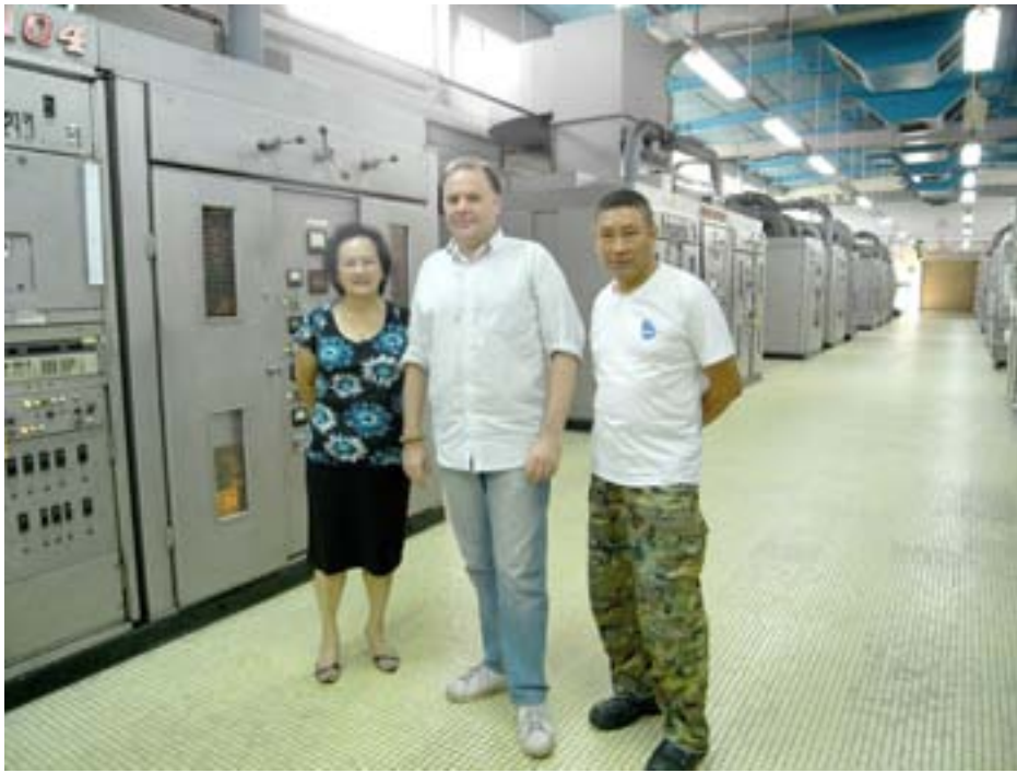
In the main transmitter hall with Cindy Yao, the manager of the station, the author and Tam Lam Soon, the chief engineer who has been with the station for over 20 years.
