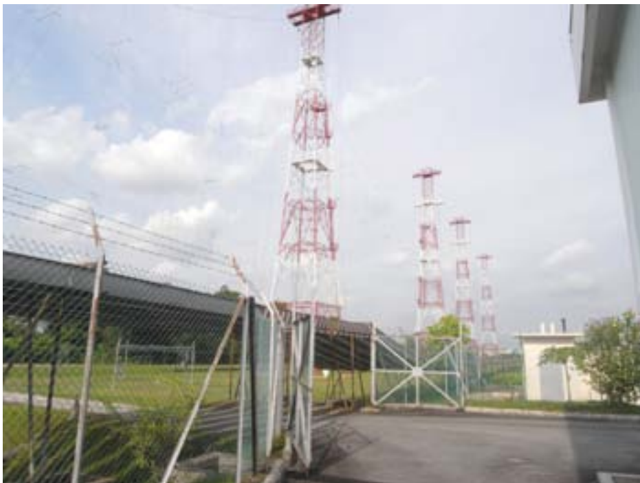
Massive BBC Far East Relay Station curtain array dominates the landscape.
