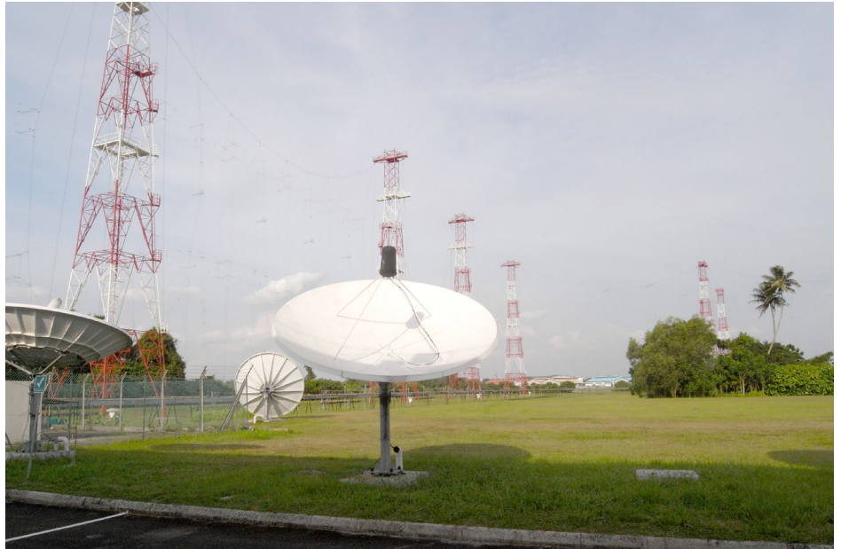
Satellite dishes to downlink BBC programming are in the foreground with the shortwave curtain antenna in the background. Note the elevation of the dishes are nearly straight up this close to the equator.
