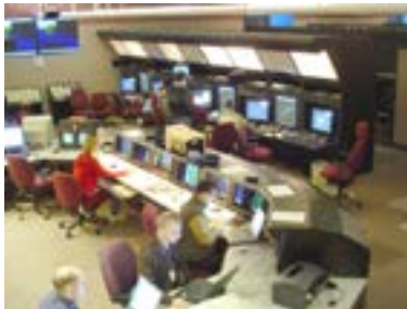
FAA ARTCC Control Room (Courtesy FAA)
