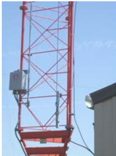
One of the WOR-710 towers, showing the wiring necessary for the aircraft warning lights. (Doug Smith)
